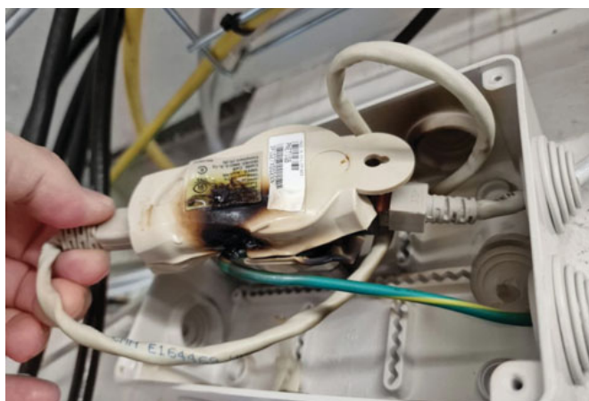
Blitzschaden am Schellenberg-Relais
